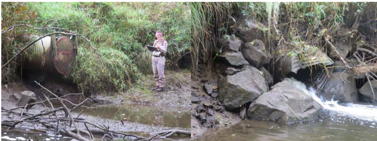
Two tidegates present on westside of Bain Slough, one still appears to be functioning (left), one has been damaged and is only a culvert at this point.
